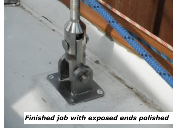
New plates with old hardware
